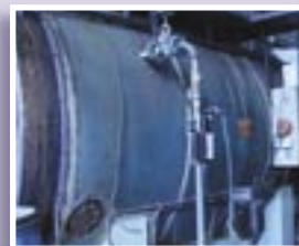
Batu Pahat Garment Industries (Malaysia): 6 Tons Steam Boiler.
