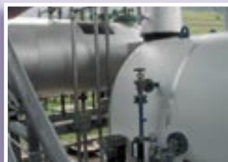
TKO Landfills Site (Hong Kong): 8 Tons Steam Boiler.
