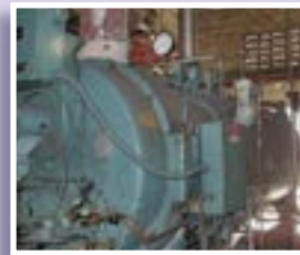
Gelmart Industrial Factory (Philippines, Manila): 4 Tons Steam Boiler
